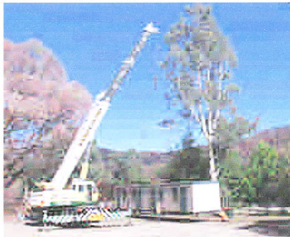
The first of the temporary Chalets being placed on the ESA site
